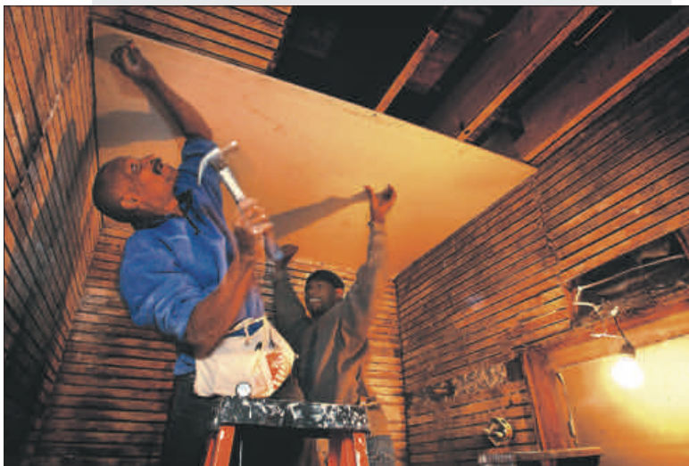
Clyde Adams and Dwayne Khaton hang drywall for the Walnut Way Conservation Corp. in what will become a new cultural center on N. 17th St. The 1907 building had been a boarding house for Southern migrants and deteriorated into a drug house. In its next life, it will house a library, archives, literacy center, computer lab and a pottery kiln.
