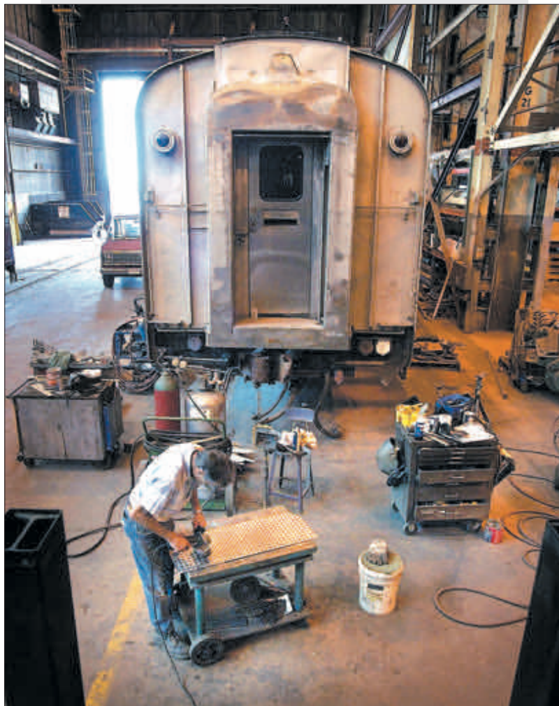
Roger Otto works at reconditioning an old train car in what was an Allis-Chalmers shipping building, where turbines were loaded onto train cars. Otto used to work for Allis-Chalmers, which was one of Milwaukee's largest employers, and now works in the same building for Avalon Rail, which restores and customizes rail cars in West Allis.
